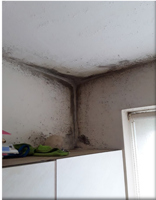
Image 3. Typical result of a kitchen not fitted with intermittent extract fans which removes moist air to the outside air.
