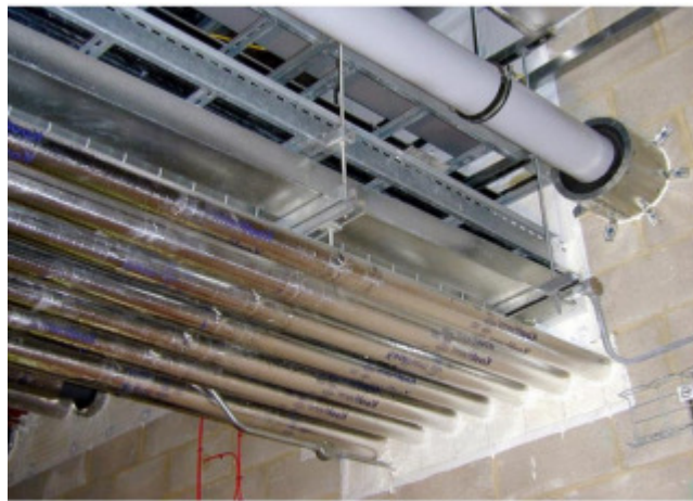
Image : Penetration of cable trays and pipes properly fire-stopped with approved materials in a fire resisting masonry compartment wall
