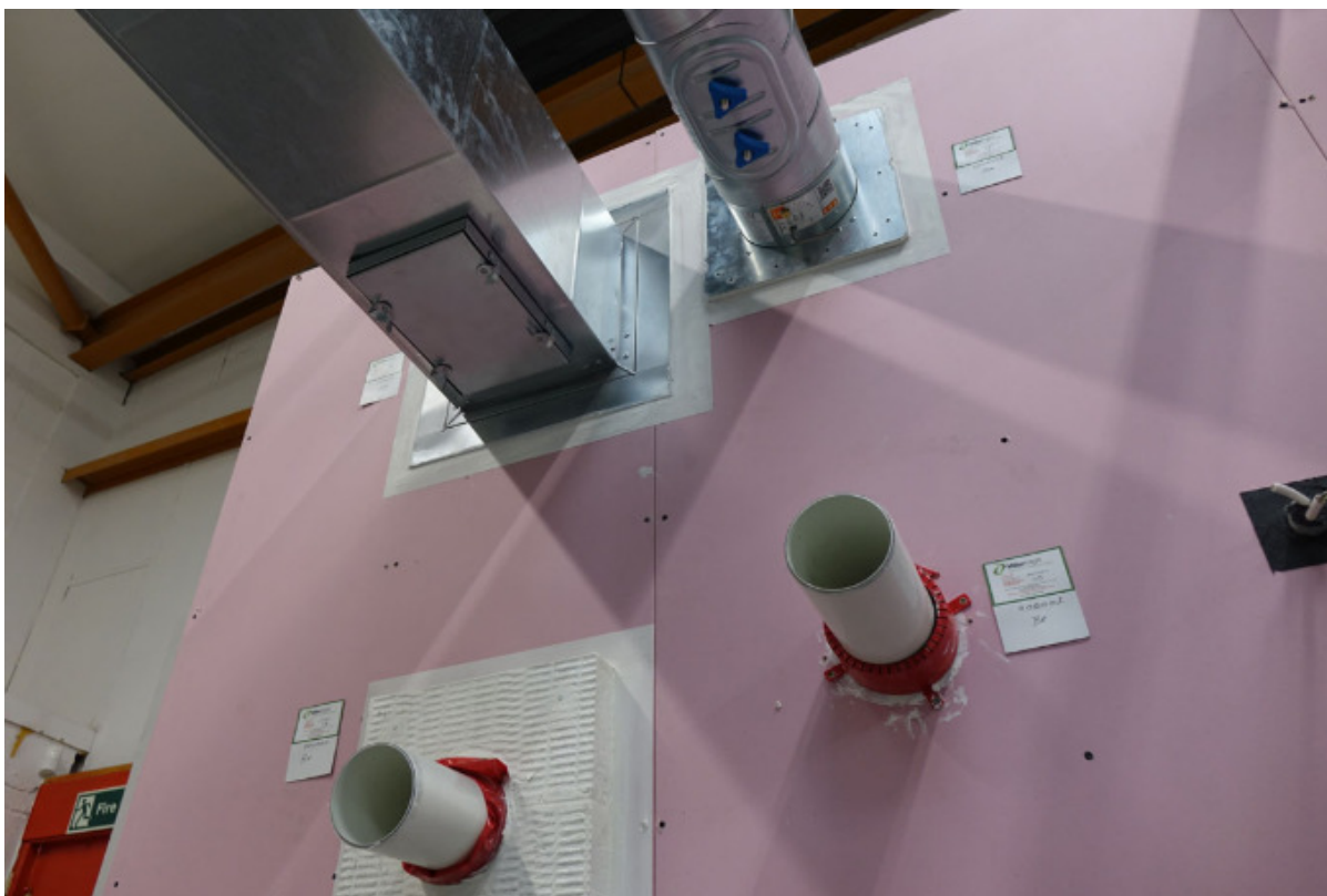
Image 2 : Showing professionally installed fire dampers on ductwork, fire collars around pipe penetrations, collars around cables – Image from HASMAN LIMITED
