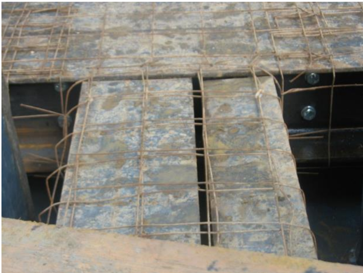
Image 1 - Typical example : Un-painted steel beams positioned in the ground, wrapped in structural D49 mesh
